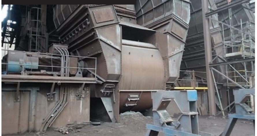
A large steelworks fan on a concrete foundation
