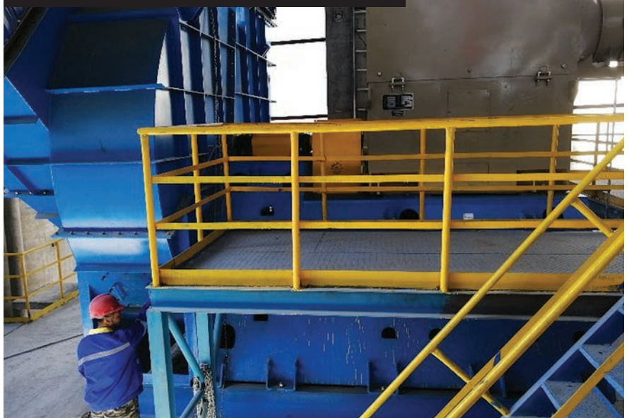
Large cement fan on the floor using anti-vibration mounts
